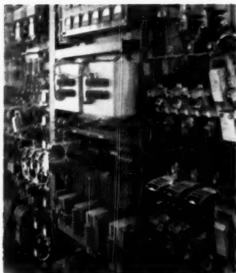
Westinghouse Load-O-Matic hoist control panel for this 125-hp, 25-cycle installation.
